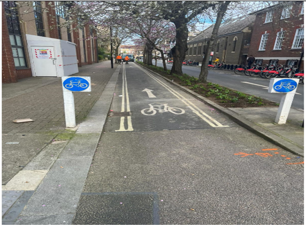
Figure 29: Crisp Walk, a healthy street – urban greening project, depaving a segregated island
